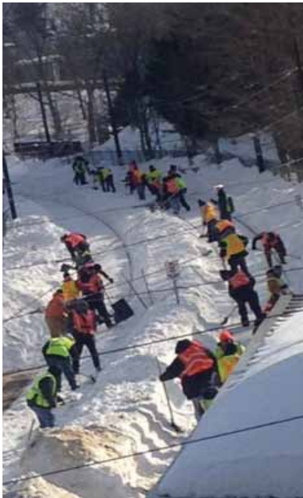
Workers labored to clear the Mattapan Trolley tracks near Milton Station over the weekend. Service resumed on the trolley line on Monday after weeks of being off-line due to snow and ice. Photo courtesy Ellen Berlin
