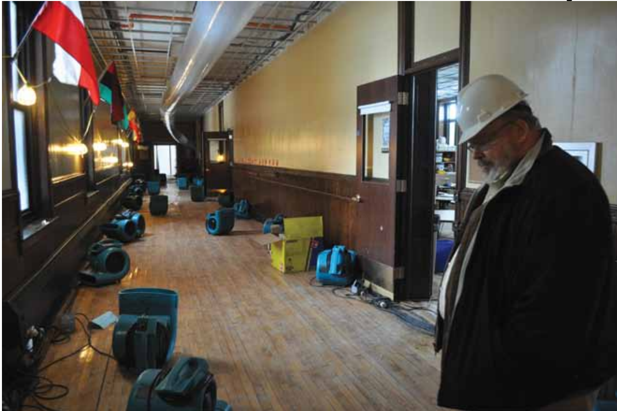
Rev. Jack Ahern surveyed the damage on the second floor of St. John Paul II Catholic Academy's Columbia campus on Monday morning. Bill Forry photo
