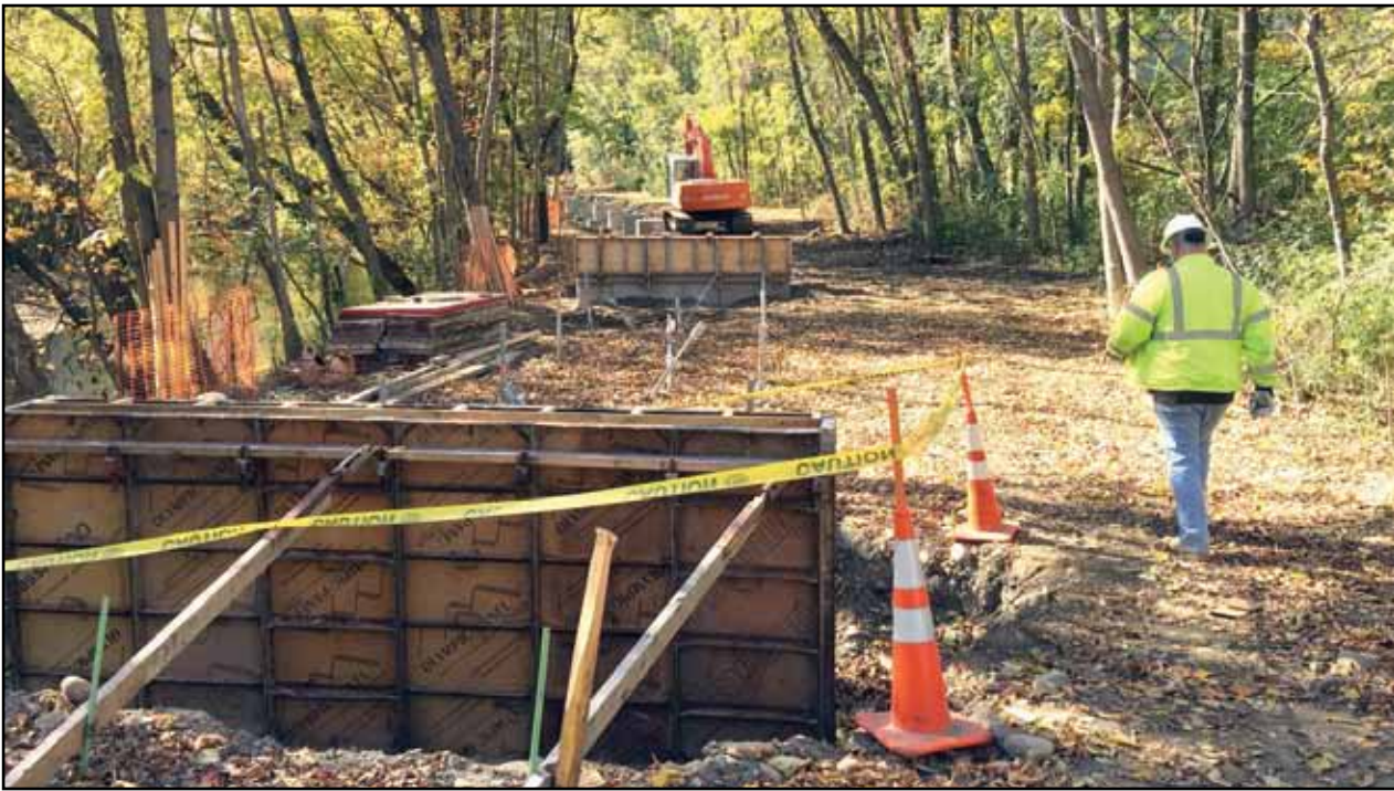
Work is proceeding this fall on a 1.3 mile extension of the Neponset River Greenway. Above, a Department of Conservation and Recreation supervisor walked along the trail on the Mattapan side of the Neponset River on Monday. The $14 million segment will be completed next spring, according to current projections. Jennifer Smith photo
