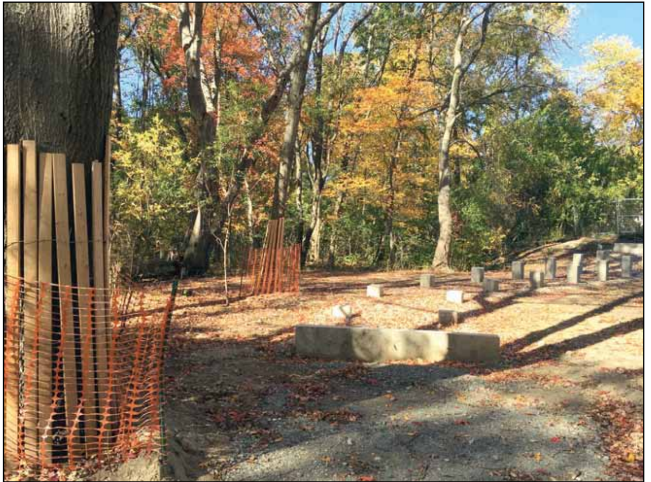
Pilings are in place for a raised wooden walkway that will lead from an existing parking lot next to Ryan Playground on River Street.
