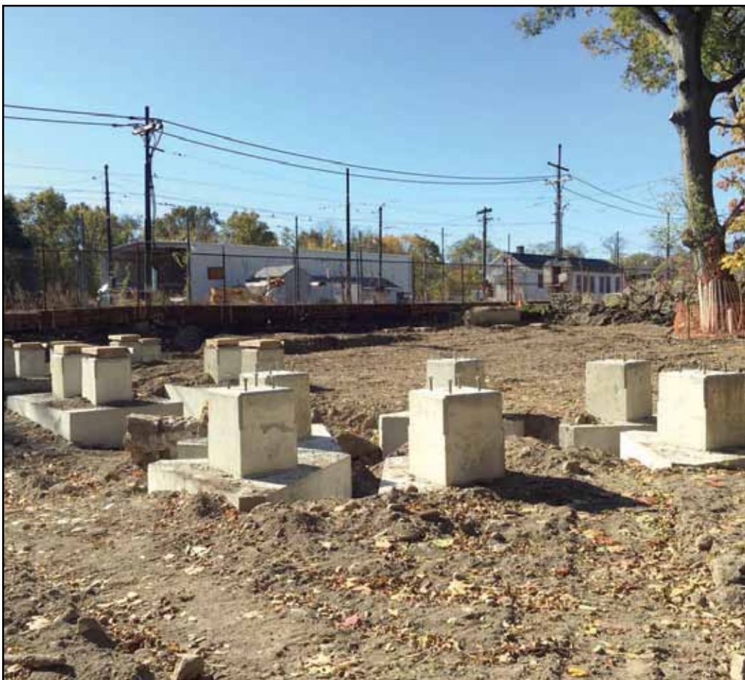
Pilings that will support a raised walkway lead to what will be a canopy bridge over the MBTA trolley tracks near Mattapan Square.
