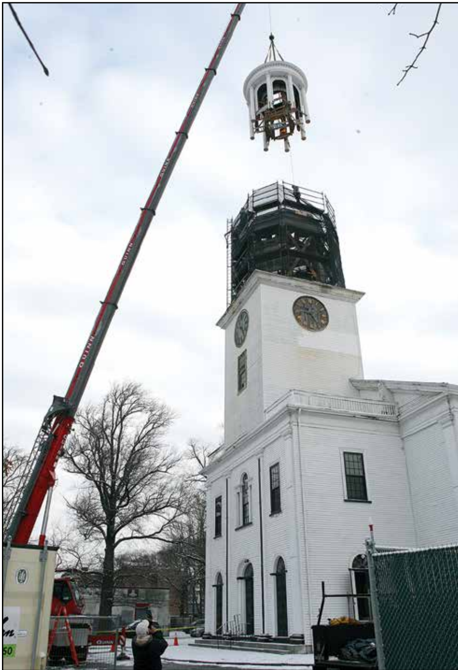
The lantern tower on the Second Church in Dorchester was lifted back in place on Jan. 29 after being repaired and sitting on the ground for the last 18 months. Other parts of the steeple will gradually be restored over the next few months. Successive projects coming very soon include restoring the clock and getting the historic Paul Revere bell ringing again. Seth Daniel photo
