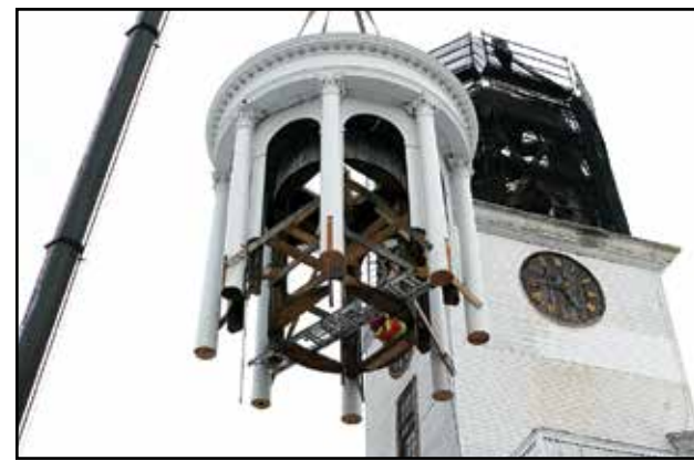
The lantern tower on the Second Church in Dorchester was lifted back in place on Jan. 29.
