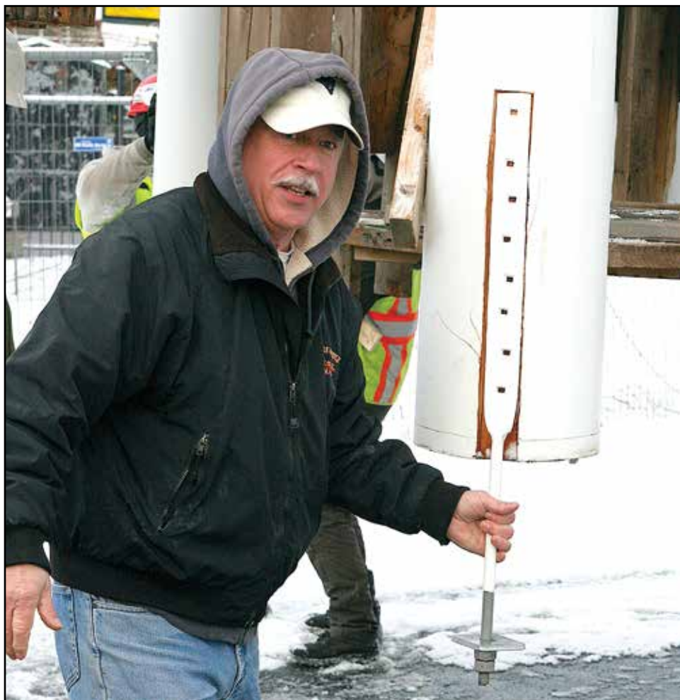
Bob Levesque, of American Steeple & Tower Co., shows the hardware that will attach the lantern tower to the steeple once it's in place. Seth Daniel photo
