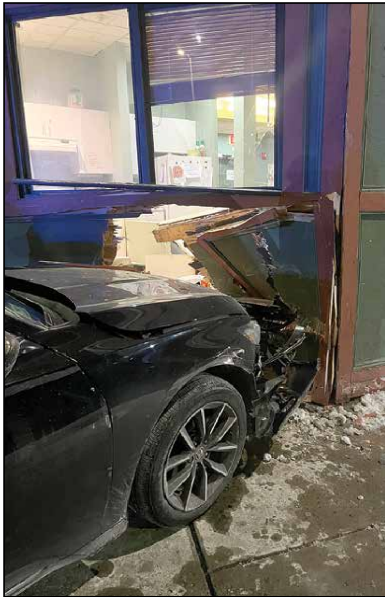
This image shows the aftermath at Ashmont Nursery School after a man crashed his vehicle into the side of the building on Washington Street. Photo courtesy ANS
