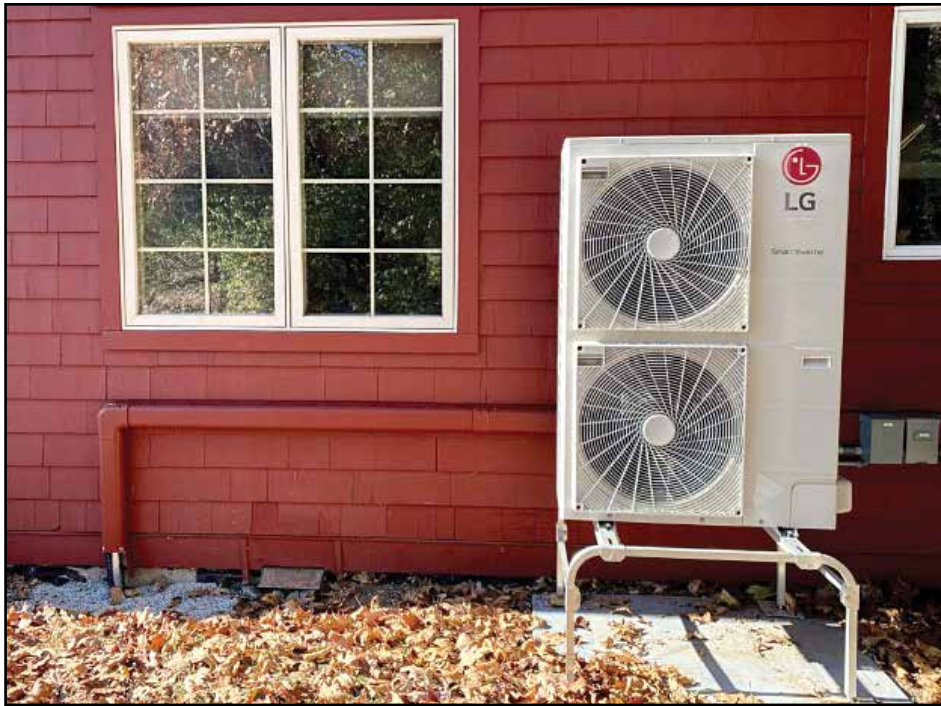
A heat pump condenser outside of a building in Lincoln, Mass.
