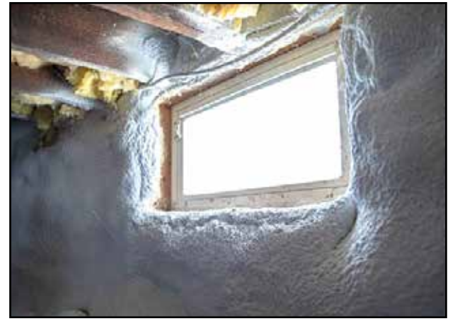
The basement wall in a renovated three-decker, where an old stone wall has been covered with a hard layer of foam insulation.
