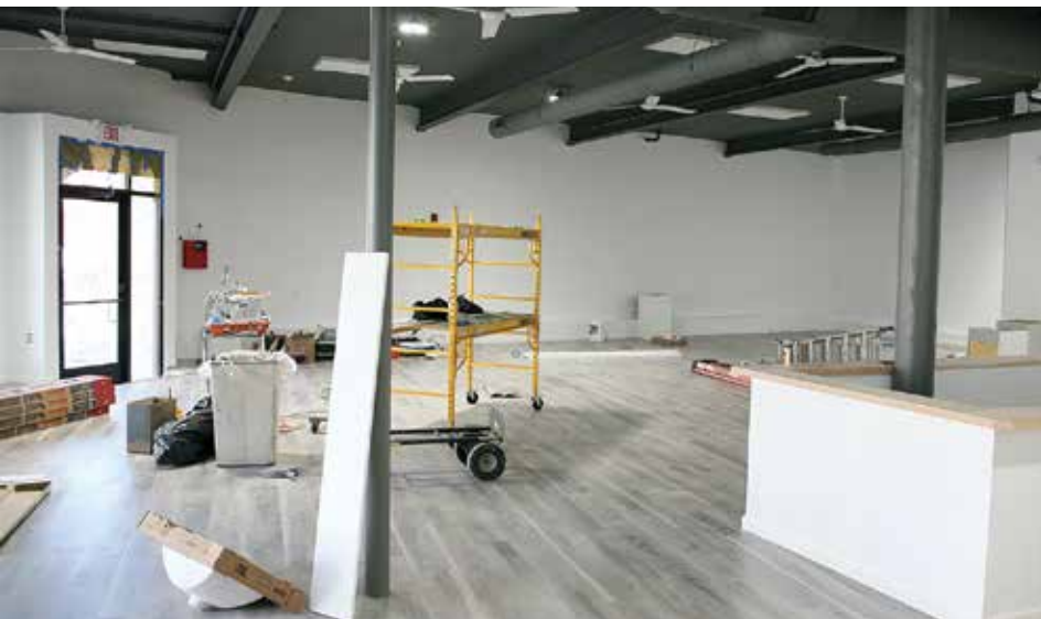
The inside of what will be the Fun Time Academy Day Care space at 9 Bowdoin St. that is expected to open in early 2025. Seth Daniel photos
