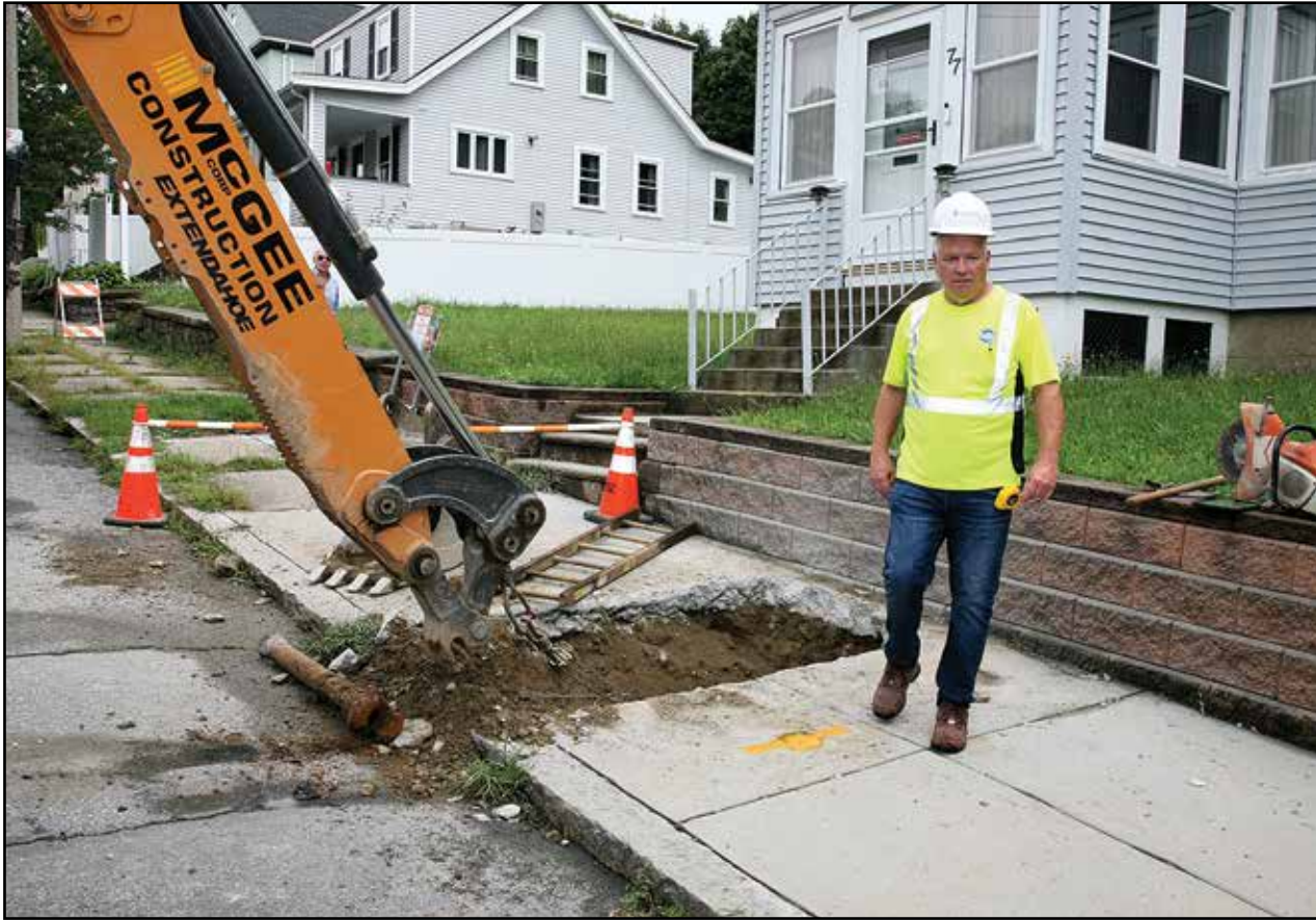
Joe Joyce, of BWSC, supervised the job on Standard Street as the team got ready to pull the lead line out of the ground. Seth Daniel photos
