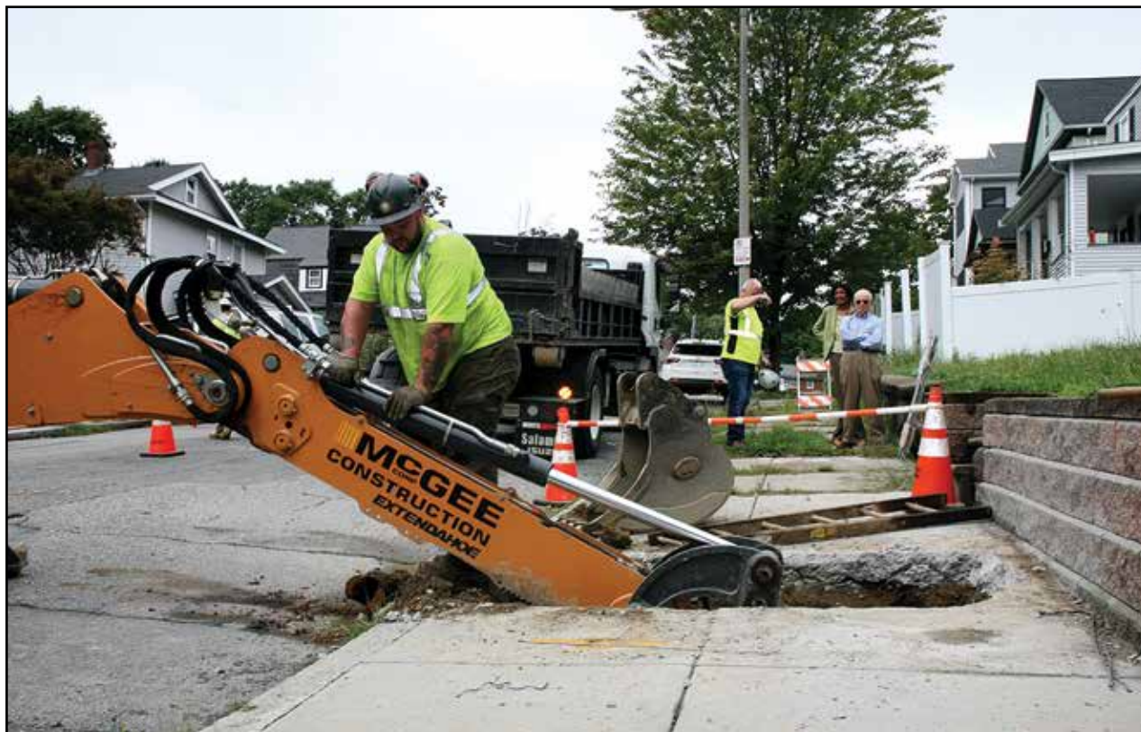
Workers positioned machinery to pull out a lead service line on Standard Street in late August while they pulled through a new copper service line from the basement of the home. Most jobs only take a few hours and, due to federal and state funding, are now free to the customer. Seth Daniel photos
