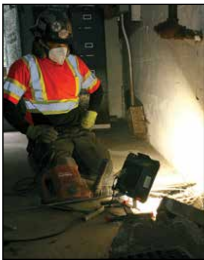
A worker from the Boston Water and Sewer Commission's lead service line replacement team prepared a lead pipe for removal from a basement in Mattapan's Standard Street in late August while guiding in the new copper line that will replace it.
