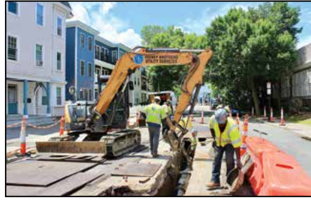
A crew worked on a trench along Savin Hill Avenue on Monday as part of an Eversource-related project. Cassidy McNeeley photo
